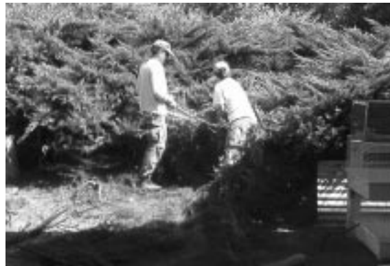
Volunteers Larry Dudus and Gerry Streff removing 8-foot-high junipers to install exercise run.
